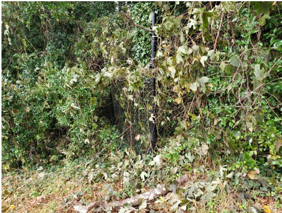
2. View of section of chain link fence that is covered by large amounts of vegetation.
