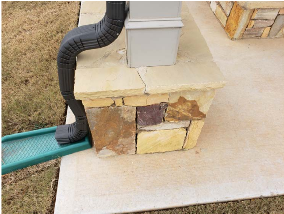
16. View of cracked stone at column of mail kiosk.
