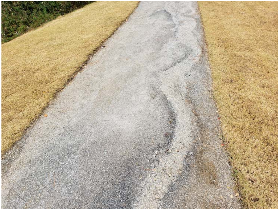
8. View of erosion along the walking trail.
