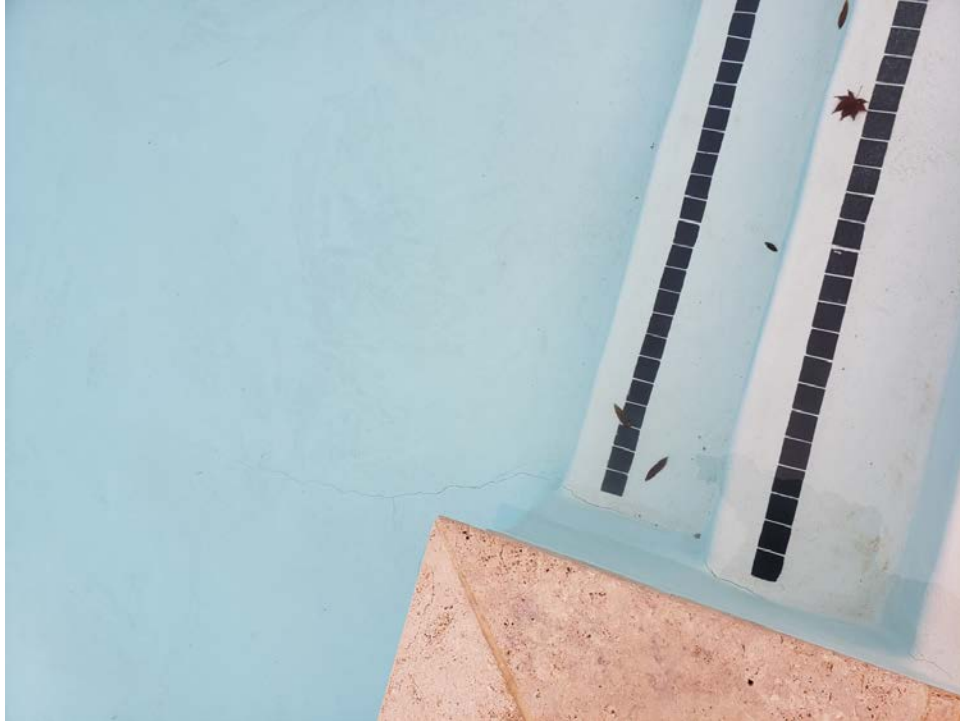
5. View of linear crack along the surface of the swimming pool.
