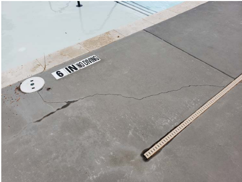
6. View of linear crack at the pool deck surface.
